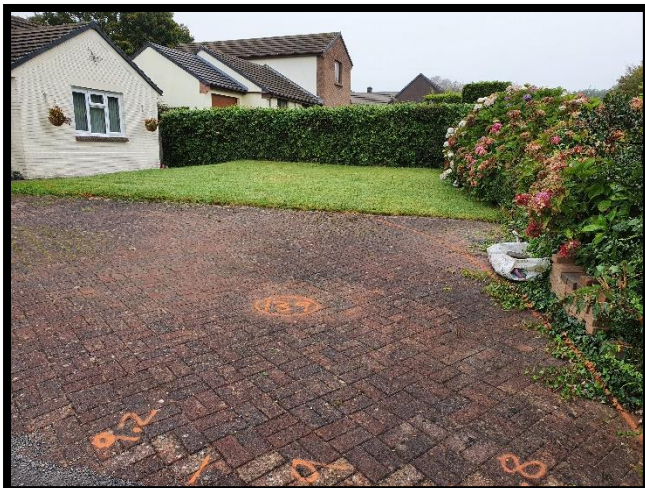
Original driveway was block paved and was looking old and tired.
